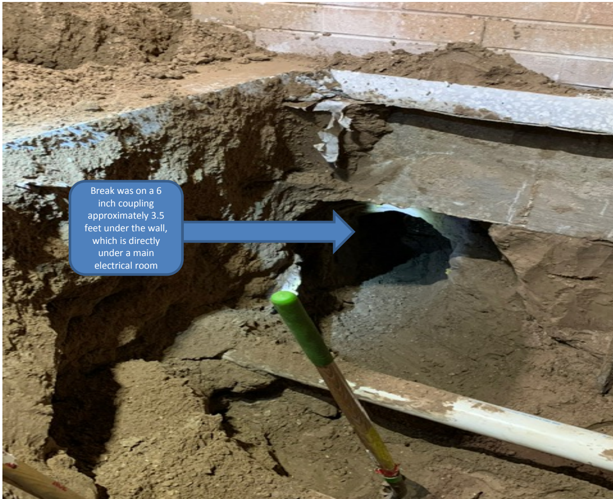
This is the third break located in the same hole out side the EVS, Med Gas Cylinder Storage rooms in the breezeway. This was a 6 inch couple located approximately 3.5 feet under the building directly under an electrical room.
